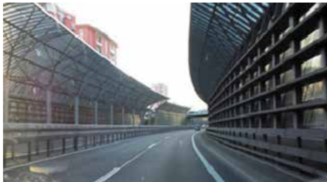
Figures 19. Noise barriers in urban area (Switzerland)
