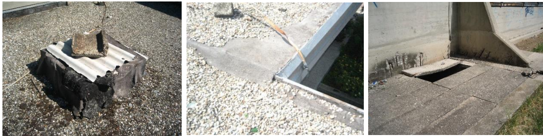
Figure 3: Damage of roof segments and façade's concrete walls
