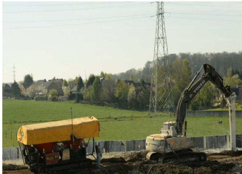
Fig. 4. Equipment used to neutralize the acid tar. On the left, the mobile feeder. On the right, the excavator equipped with the mixer.
