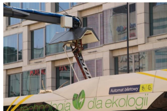
Fig. 3. Pantograph of charging system Słunik (Kraków, Poland)
