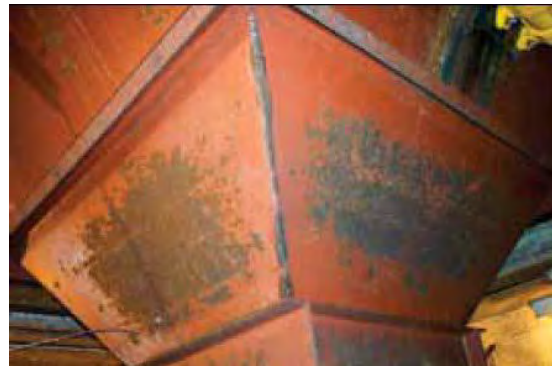
Fig. 18 Damages of the outside surface of hoppers
