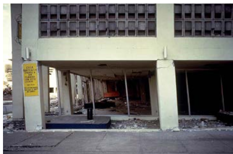
Figure 1. Soft-story mechanism in the ground floor
