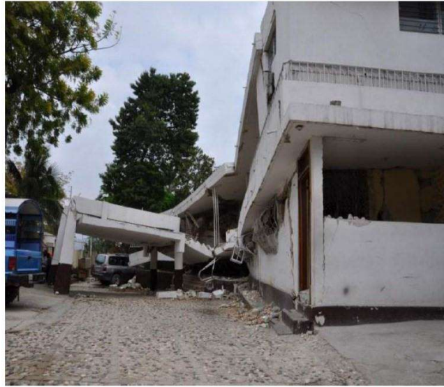
Figure 31- Damage to Ministry of Culture building during 2010 Haiti earthquake, [14]
