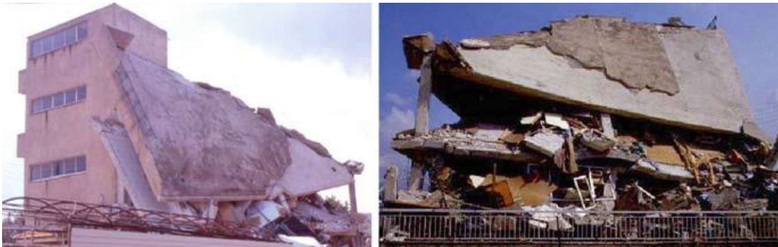
Figure 32- Collapse of a building due to torsional response, Athens (1999) earthquake
