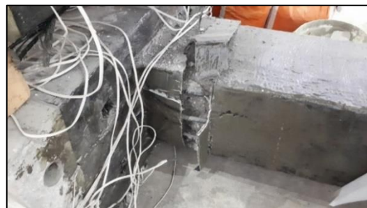
Figure 9. Observed damages during the quasi-static testing of Model M1
