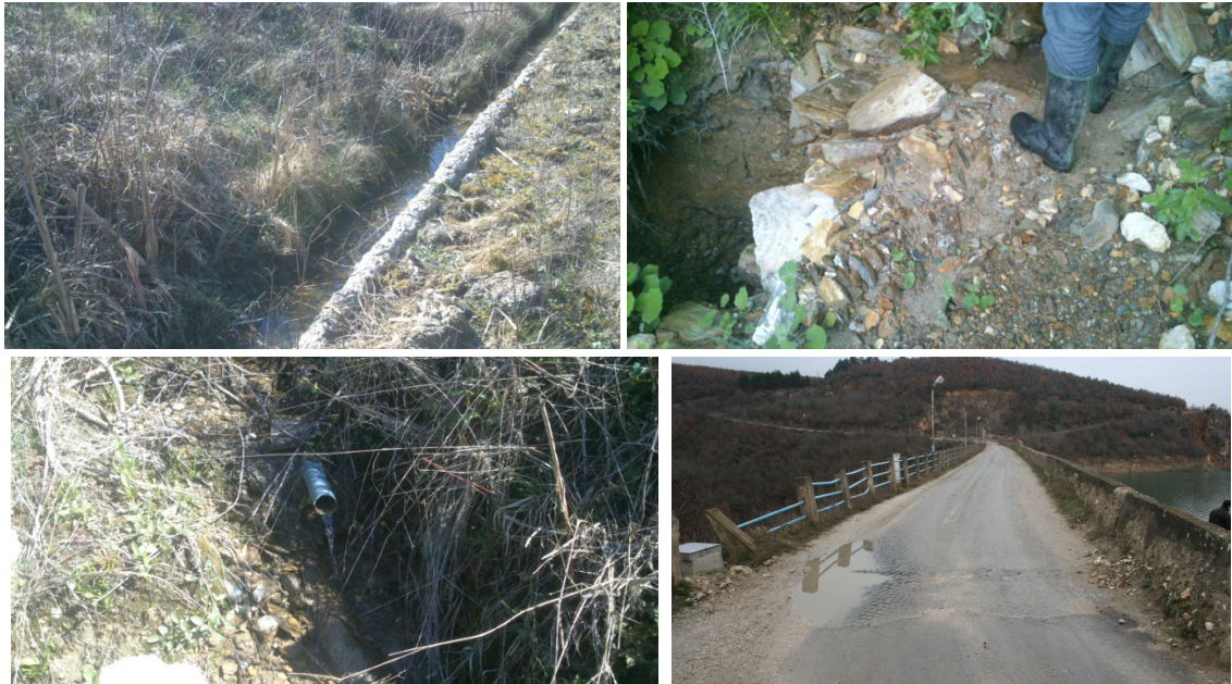
Figure 4: Wetting on the bench, gully on the right groin, sources and water retention on the dam crown.
