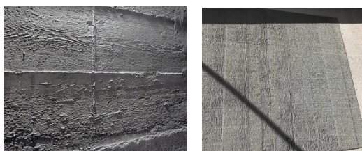
Fig.4 Old natural concrete façade, original material, before aerogel plaster (left), after aerogel plaster application (right)
