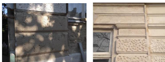
Fig.3 Old renaissance building façade [15] original material before aerogel plaster application (left); after aerogel plaster application (right)
