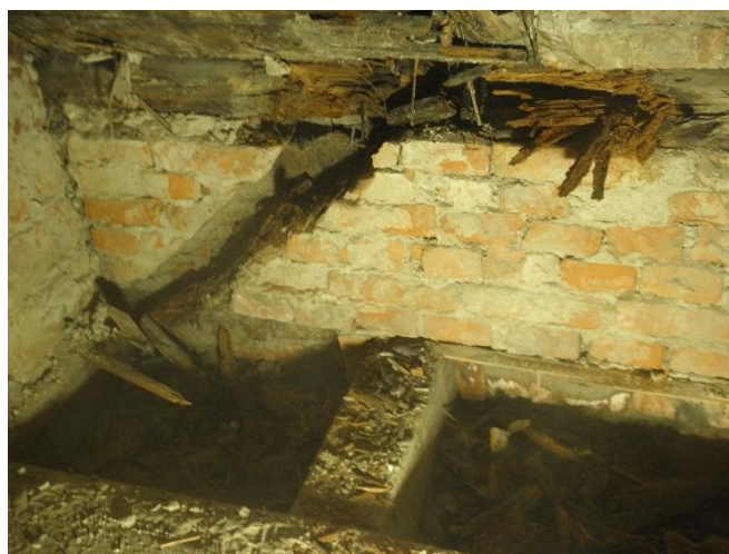
Figure 7. Visual inspection of building A – Example of a building corner with beams inserted into the wall, completely rotted.
