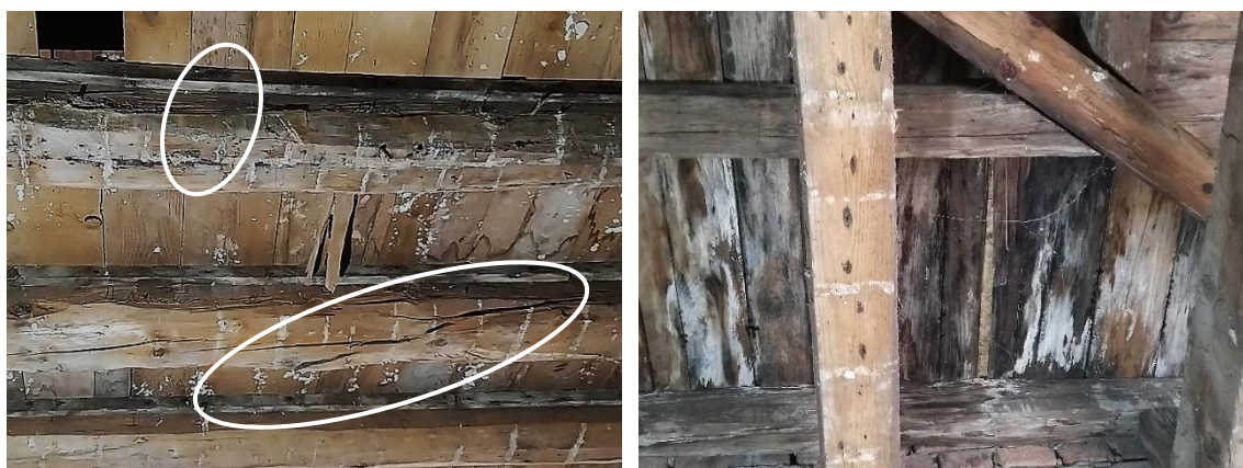
Figure 14. Attic floor beams: Left - two adjacent transversely cracked attic floor beams; Right - completely rotten beams of the northwestern part of the building
