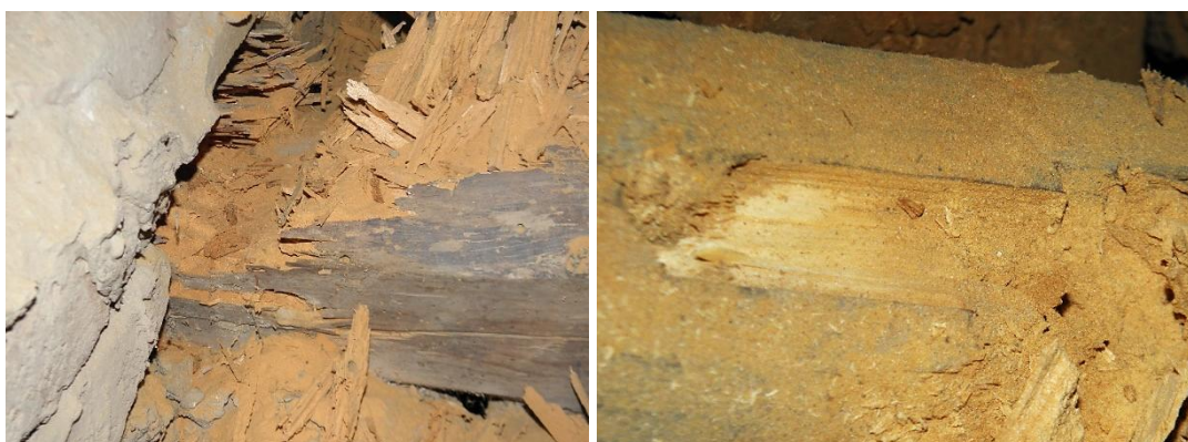
Figure 12. Beam insert in the wall: a) entire cross section decayed and degraded by insects; b) surface brown rot 12 mm in depth with sound inner part of the beam
