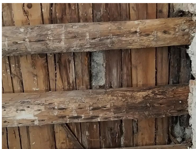
Figure 13. Severely rotten and attacked by insect beam ends inserted in north faced outer wall
