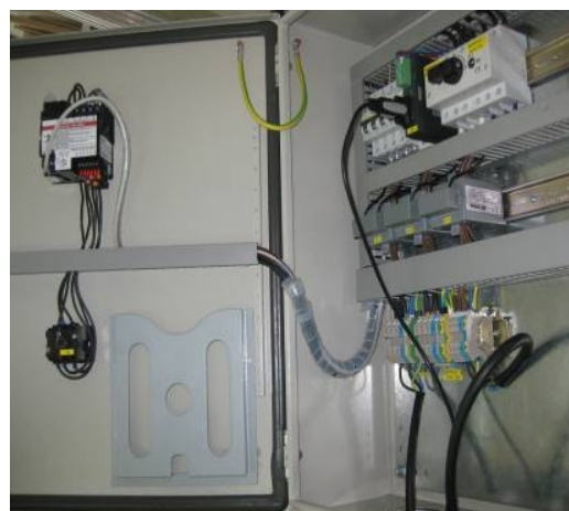
Figure 6: SRD 2 installation setup.
