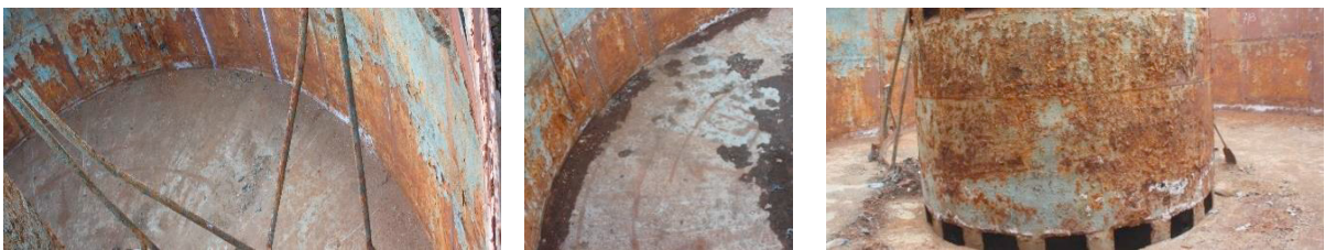
Fig. 3. Photo documentation of the current situation of the tank
