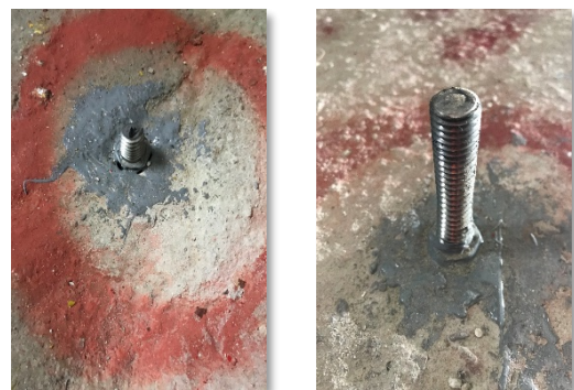
Figure 12. Failure of anchor type 4
