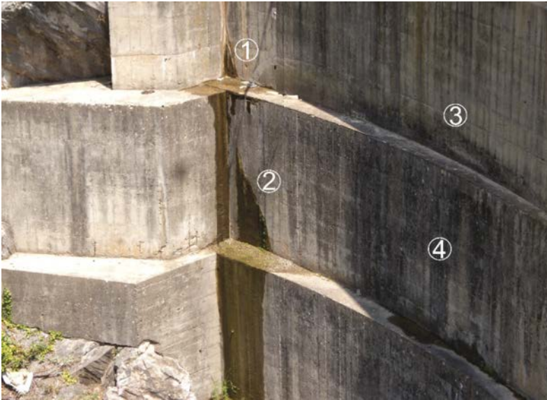
Fig. 3 Location of the cracks Emplacement des fissures
