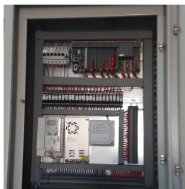
Fig. 1. IAS electrical panel
