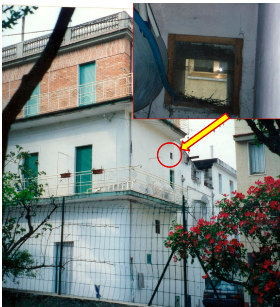
Figure 3. A pigeons' nest in close proximity to an apartment, identified during an inspection to investigate a D. gallinae outbreak (original, M.A. Cafiero).
