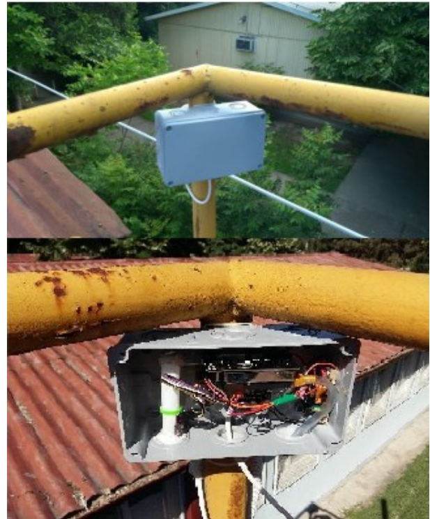
Figure 2: Sensor node box including sensors, microprocessor, Wi-Fi module
