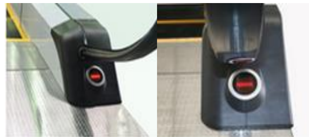
Fig. 9. Emergency stop switch
