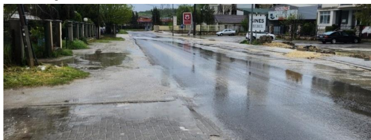
Figure 3. Inadequate drainage at km 3+200
