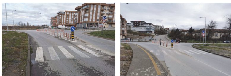
Figure 1 Existing solution of the intersection – view from both sides of street Partizanska [source: Author]
