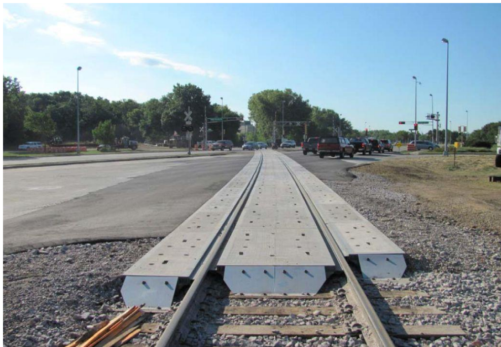
Figure 8. Example of a crossing with concrete panels in the USA (Highway-Rail Grade Crossing Surface Material Performance, NURail Research Project, 2010)
