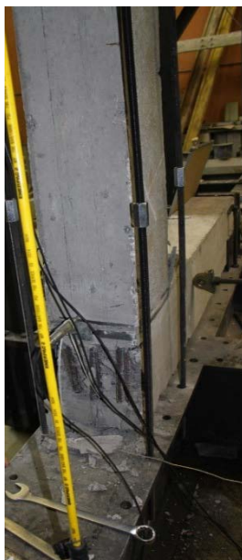
Fig.5.14. Concrete spalling in specimen "S 2, V.D." due to rotation of the dowel
