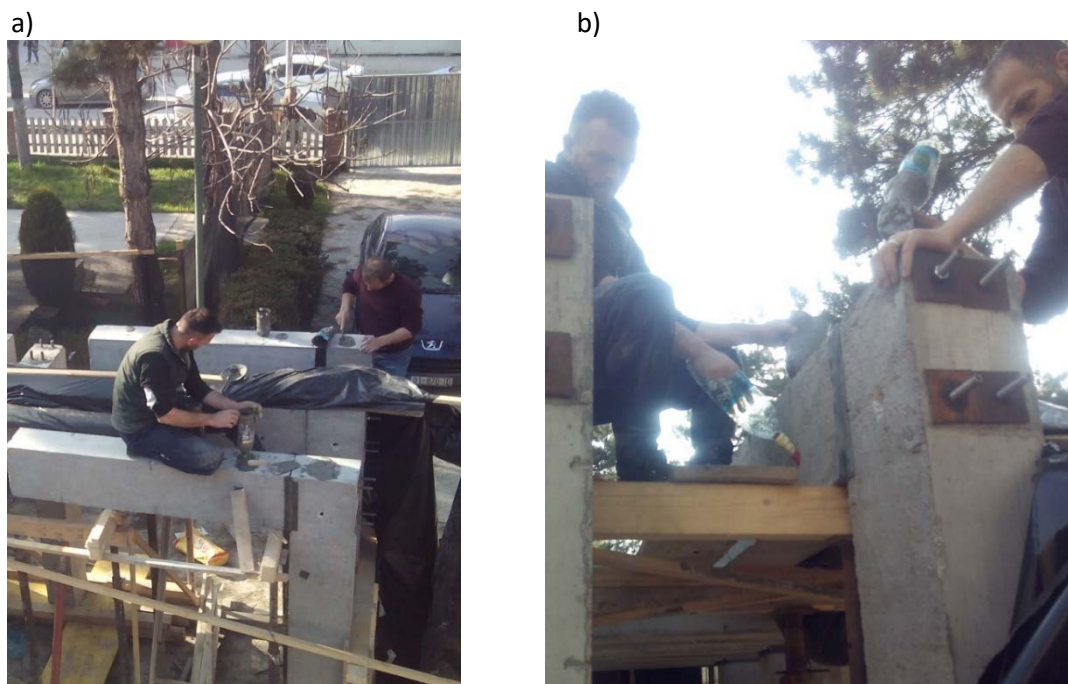
Fig. 4.21. Photo taken during performance of a connection with horizontally positioned dowels; a) filling of the upper sleeves, b) filling of the upper and the lower sleeves.
