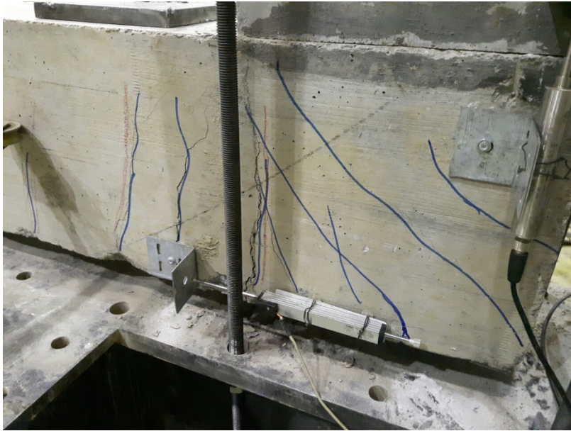
Fig. 4.32 Cracks in the specimen after the sixth loading cycle applied on specimen "S.1 V.D."
