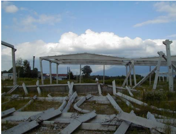
Fig. 2.9. Collapsed industrial building near Adapazari – Turkey. Failure occurred at the connection, mostly at beam-to-column connections.
