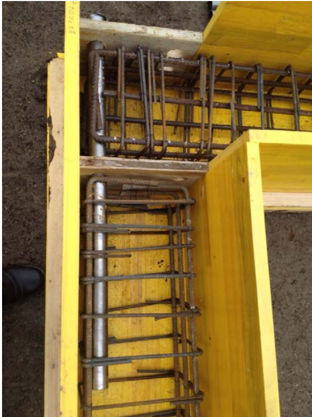
Fig. 4.19. Photo taken during construction of elements with horizontally positioned dowel, a steel pipe being inserted for sleeve preservation.
