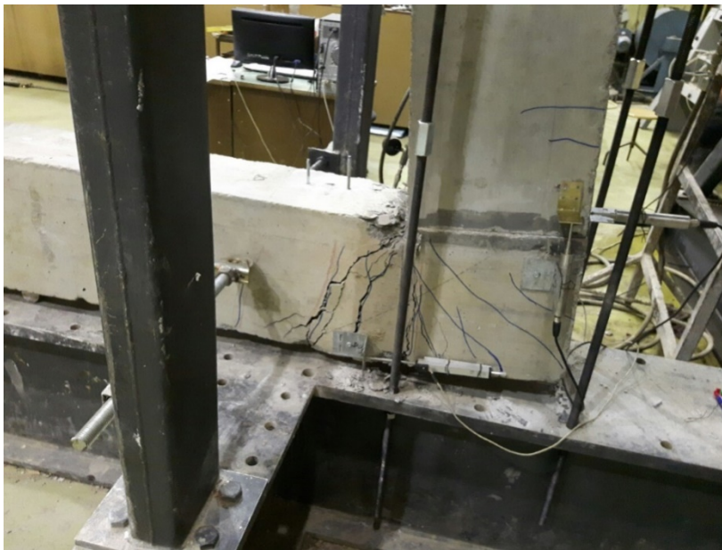
Fig. 4.33 The specimen after the last loading cycle, failure state of specimen "S.1 V.D."
