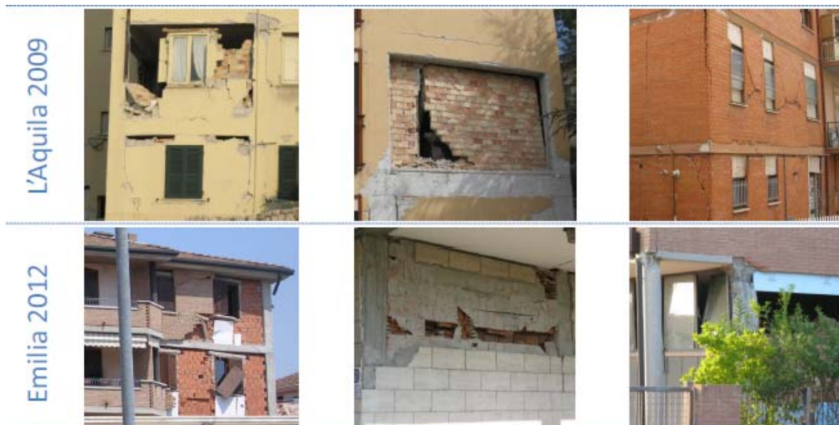
Figure 3. 1 Damages on infill walls (Photos: L.D. Decanini & L. Liberatore, L’Áquila EQ, 2009; R. Milanesi, P. Morandi, G. Magenes & B. Binici, Emilia EQ, 2012)
