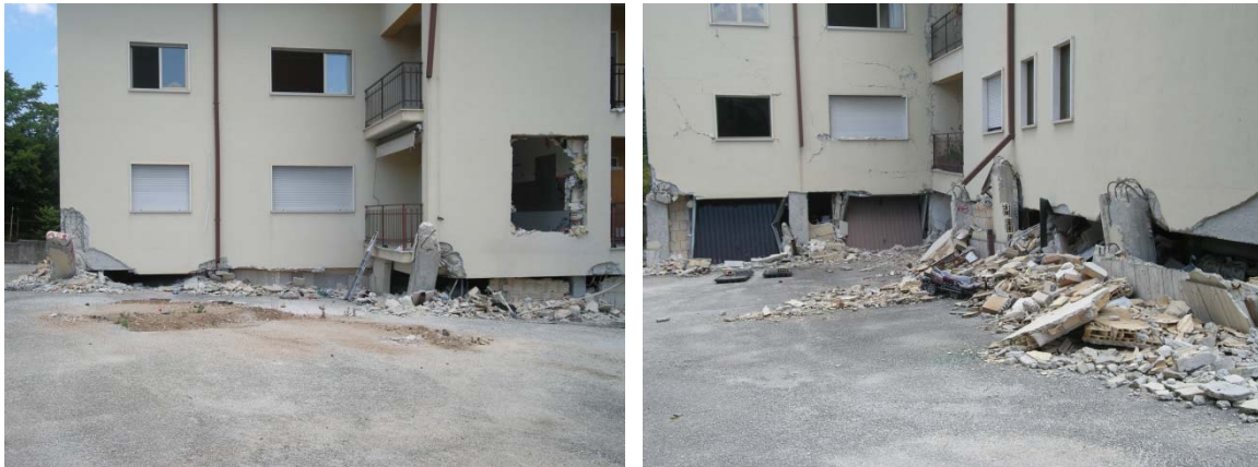
Figure 3. 2 Negative effect of infill on seismic performance of structure – “soft storey” mechanism (Photos: L.D. Decanini & L. Liberatore, L’Áquila EQ, 2009)
