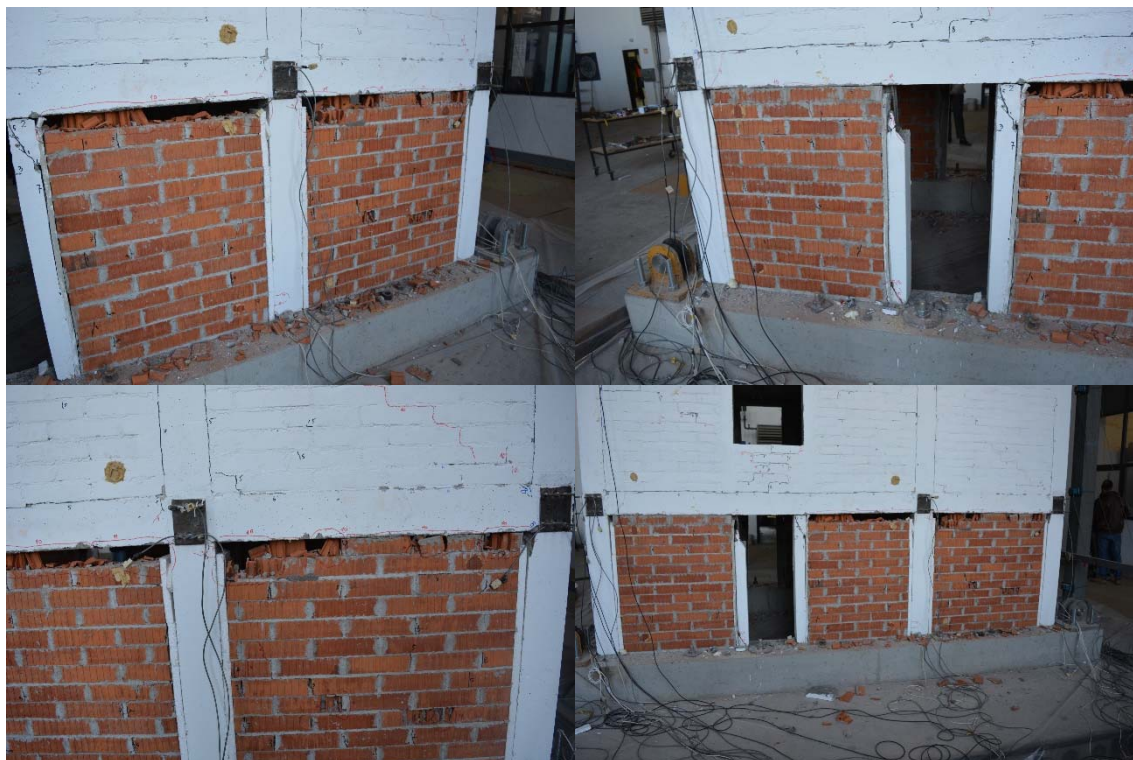
Figure 4.30 Damage to infill of the Model IW-SB -frame B- infill connection - second variant solution
