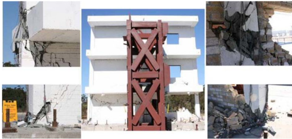
Figure 3. 9 Pictures of damaged specimen and column failure in the first storey after tests (Stavridis and Shing, 2012)
