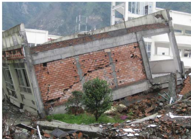
Figure 1.1 Collapse of a two-storey infilled RC building during the 2008 Wenchuan earthquake (Photo creator: Zhe Wang) (Zhang, 2015)
