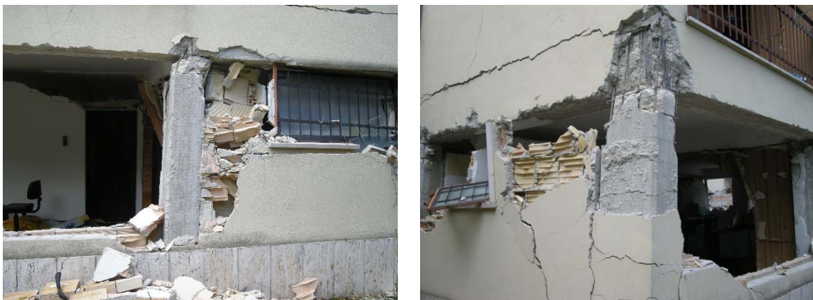
Figure 3. 3 Negative effect of infill on seismic performance of structure (Photos: L.D. Decanini & L. Liberatore, L’Áquila EQ, 2009)
