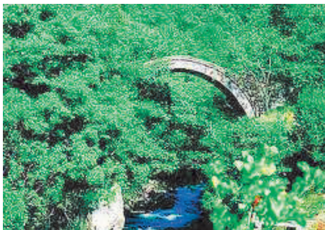
Figure 14. Stone bridge Elenski skok on Garska river (16 th century) (Nikolovski and Ivanov, 2013).
