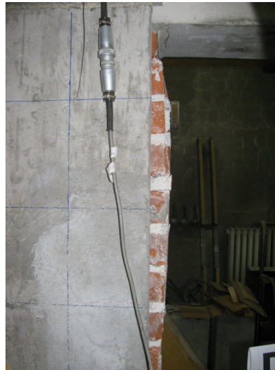
(d) Squeezing of encased masonry wall from RC jackets
