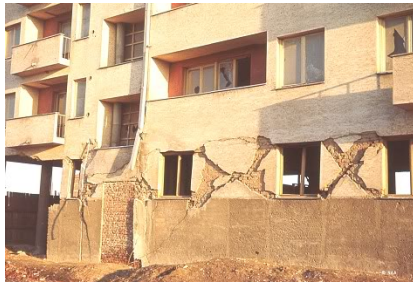
(a) In-plane damage on residential masonry building after 1963 Skopje earthquake [Ambraseys, 1967]
