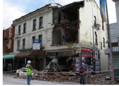
(b) Out-of-plane failure of walls after 2010 Canterbury earthquake [Ing-ham and Griffith, 2011]
