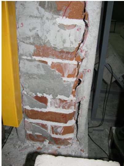
(c) Separation of RC jackets from masonry walls
