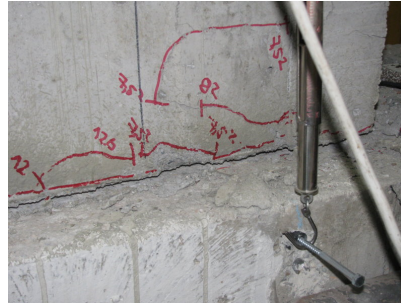
(b) Horizontal crack between the bottom RC beam and the wall and uplifting of the wall
