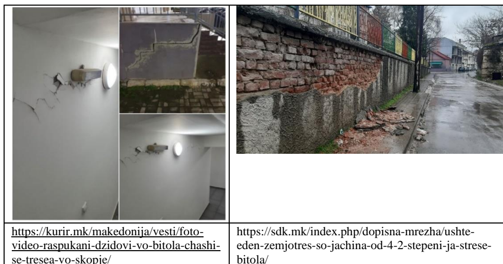
Figure 3. Damage caused by the earthquake on January 9, 2022 at 21h 43min (UTC) with local Richter magnitude M_L = 5.6 , intensity I = V-VI degrees according to the European Macroseismic Scale (EMS-98).
