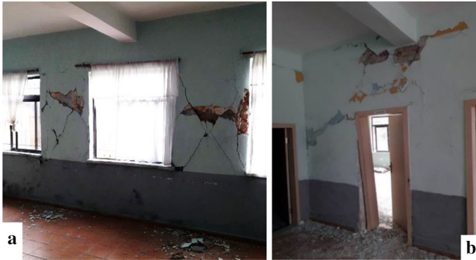
Fig. 15 Damages in school building GF+ 1 (combined system of solid brick masonry and RC elements): a diagonal cracks between the windows; b cracks in the beam supporting area
