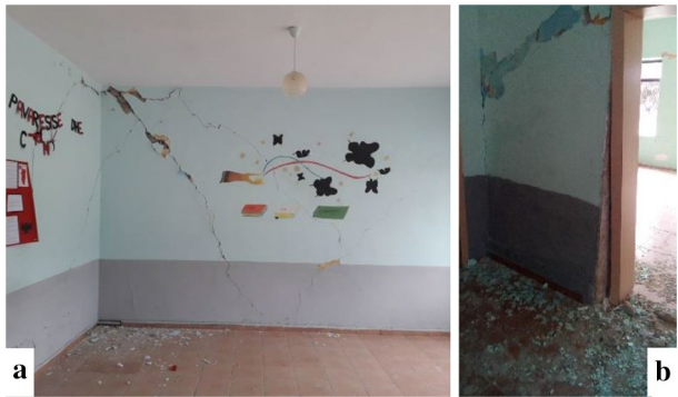
Fig. 16 Damages in school building GF+ 1 (solid brick masonry system)-diagonal cracks in brick walls. a facade wall; b infill wall
