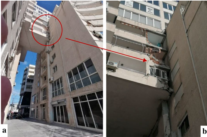
Fig. 21 Damaged bridge between two buildings located on the higher level (Grade 4). Warm connection of bridge between two buildings with undefined dynamic response
