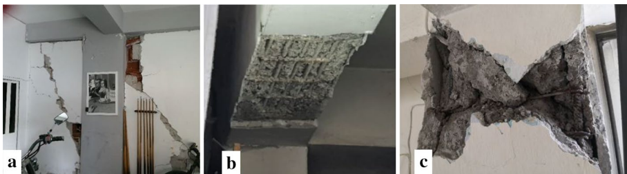
Fig. 20 Residential RC building with severe non-structural and slight structural damages (Grade 3). a Diagonal cracks in infill walls b destroyed cover layer in beam c damage in columns
