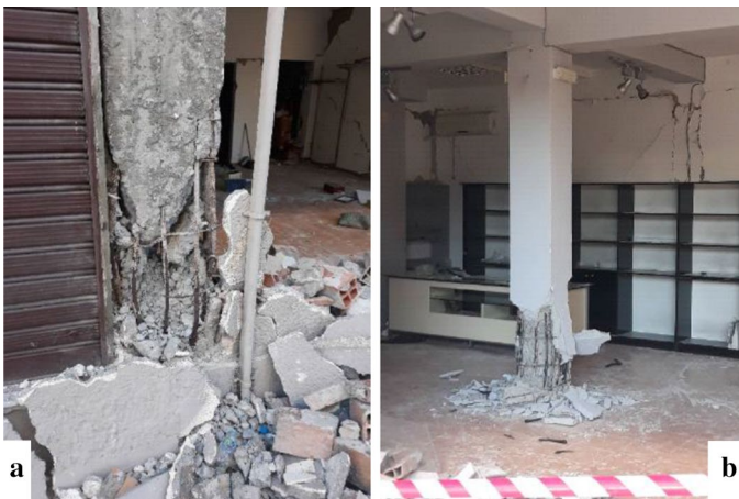
Fig. 26 Individual house GF+1. a Plastic hinges in lower part of facade column and failed facade wall b plastic hinge in middle column and separation of structural with non-structural elements
