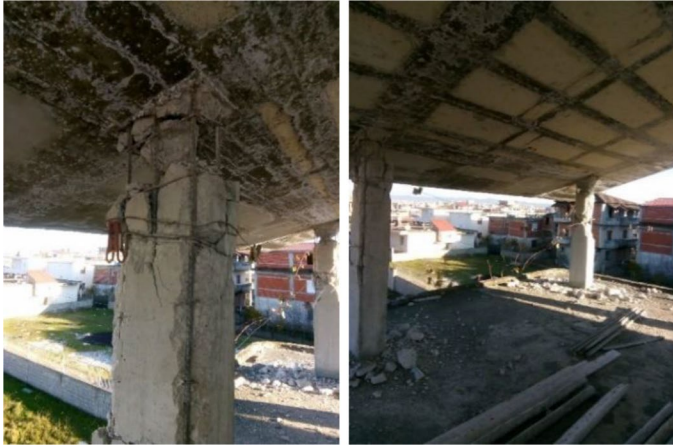
Fig. 25 Individual house GF+2 with plastic hinges in upper part of columns due to low quality concrete and stirrups with small diameter
