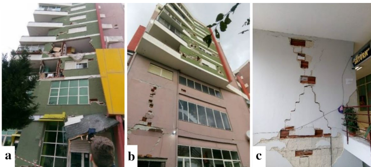
Fig. 17 Structures with major non-structural damage (Grade 3). a Failure in the front façade due to absence of belt courses; b damage of the rear façade in all levels; c shear damage emphasized with the diagonal cracks in infill wall on first floor
