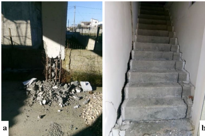
Fig. 24 Individual house GF+1 with major structural and non-structural damage due to lower quality of concrete, unsafe for habitation (Grade 5). a Plastic hinge in lower part of column; b separation of the stair structure
