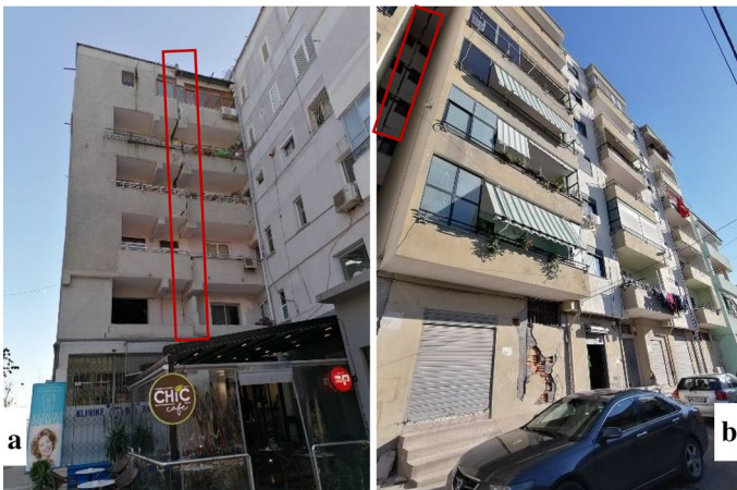
Fig. 22 Collision between two adjacent buildings (Grade 4). Expansion joint with small width
