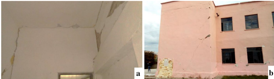
Fig. 14 Damages in school building GF+1 (combined system of solid brick masonry and RC elements): a separation of orthogonal walls; b shear damage in facade wall with diagonal cracks
