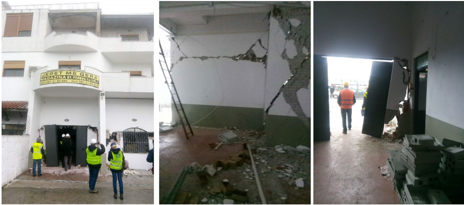
Fig. 16 Low-rise buildings with heavy structural damage to the first level after the Durres earthquake
