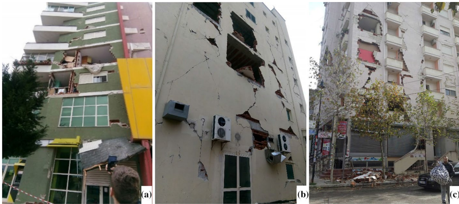
Fig. 20 Mid-rise building damaged after Durres in Albania, earthquake 2019. a and b (Sheshov et al. 2021); c ( https://www.caritas.eu/earthquakes-in-albania )
