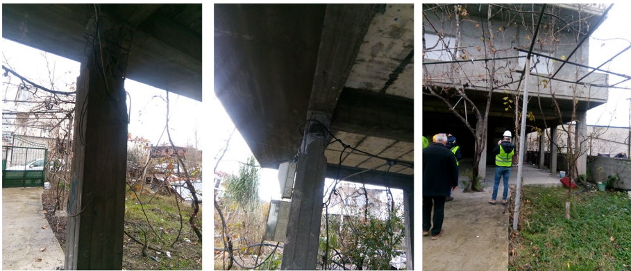
Fig. 17 Damaged columns at the ground floor of a low-rise building after the Durres earthquake
