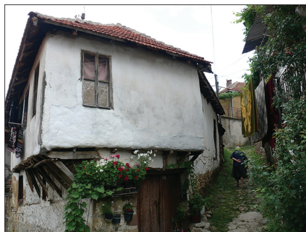
Figure 12. A solution for the triangle cantilever with wooden supporters at the corner of the house - simple and easy solution for the problem.
