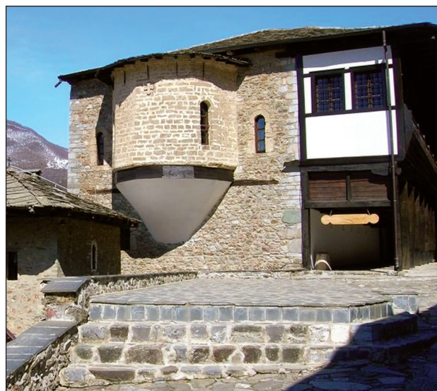
Figure 18. A rare sample of a cantilever, which can be found at searching a solution for expanded fireplaces. The example is a part of the dining room of the monastery, where the polygonal form is transformed into a cone ending. Tending to hide the wooden supporters which cross themselves unevenly, in order to create a visual statics, the cone ending is covered with mortar.
