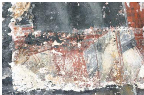
Fig. 2. Details of the two layers of paint from the 17 th (middle layer) and from the 19 th century (upper and lower layers) from one of the walls in Sv. Bogorodica Church in Lešok. (The colour can be seen on the on line Internet issue)
